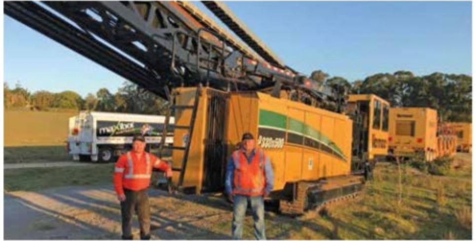
Maxibor's new rigs and the other equipment that will be required for the long bores.
