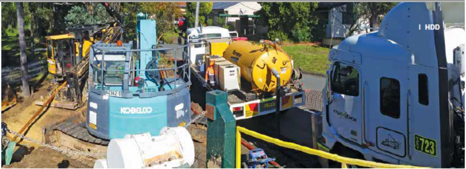
Maxibor's setup for 10 km of HDD as part of an NBN project in Toronto, NSW.
